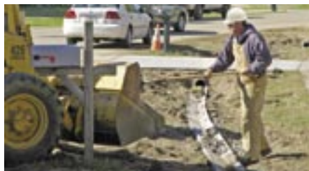
A contractor works on final restoration after installing a roadside paved swale as part of the Toebbe Lane DRI project.
