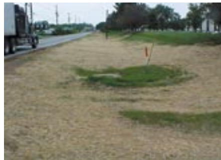
Flooding problems are resolved with drainage improvements like this construction project along Grade Lane.
