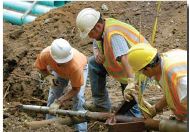
A construction crew installed a pipe under Story Avenue without excavating the roadway as part of a project to eliminate a combined sewer overflow.
