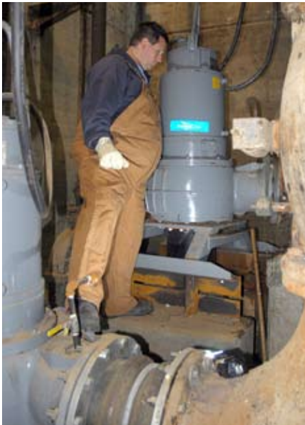
Dave Ciez inspects equipment at the Fourth Street Pumping Station.
