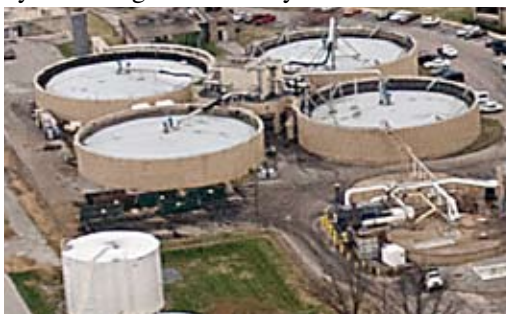
The Digester Control Building at the Morris Forman Water Quality Treatment Center will receive two condensate accumulator tanks to control the collection of condensation and decrease corrosion.
