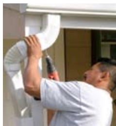
An MSD contractor disconnects a rain-gutter downspout from the sanitary sewer system.
